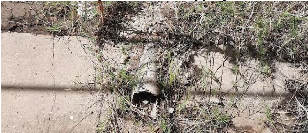
Figure 11: Asbestos based pipe exposed.
