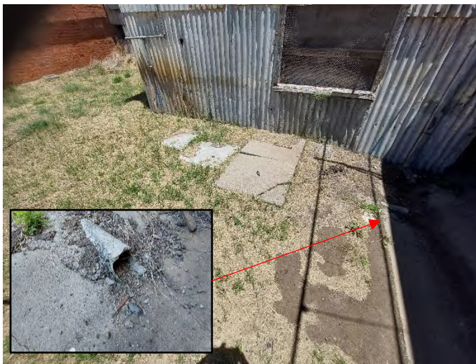
View of grease trap
