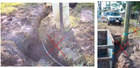
Above: Poles with become unstable if undermined
